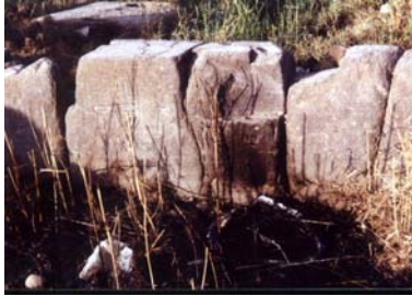
Fig. (1): Basaltic blocks highly cracked due to weathering & plant vegetation, Memphis
